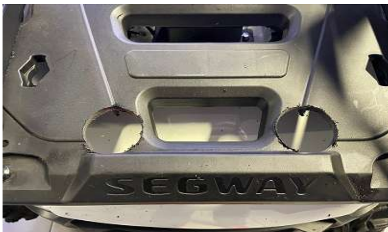
Drill holes with a crown with a diameter of 50-52mm. Then remove the rack platform.
